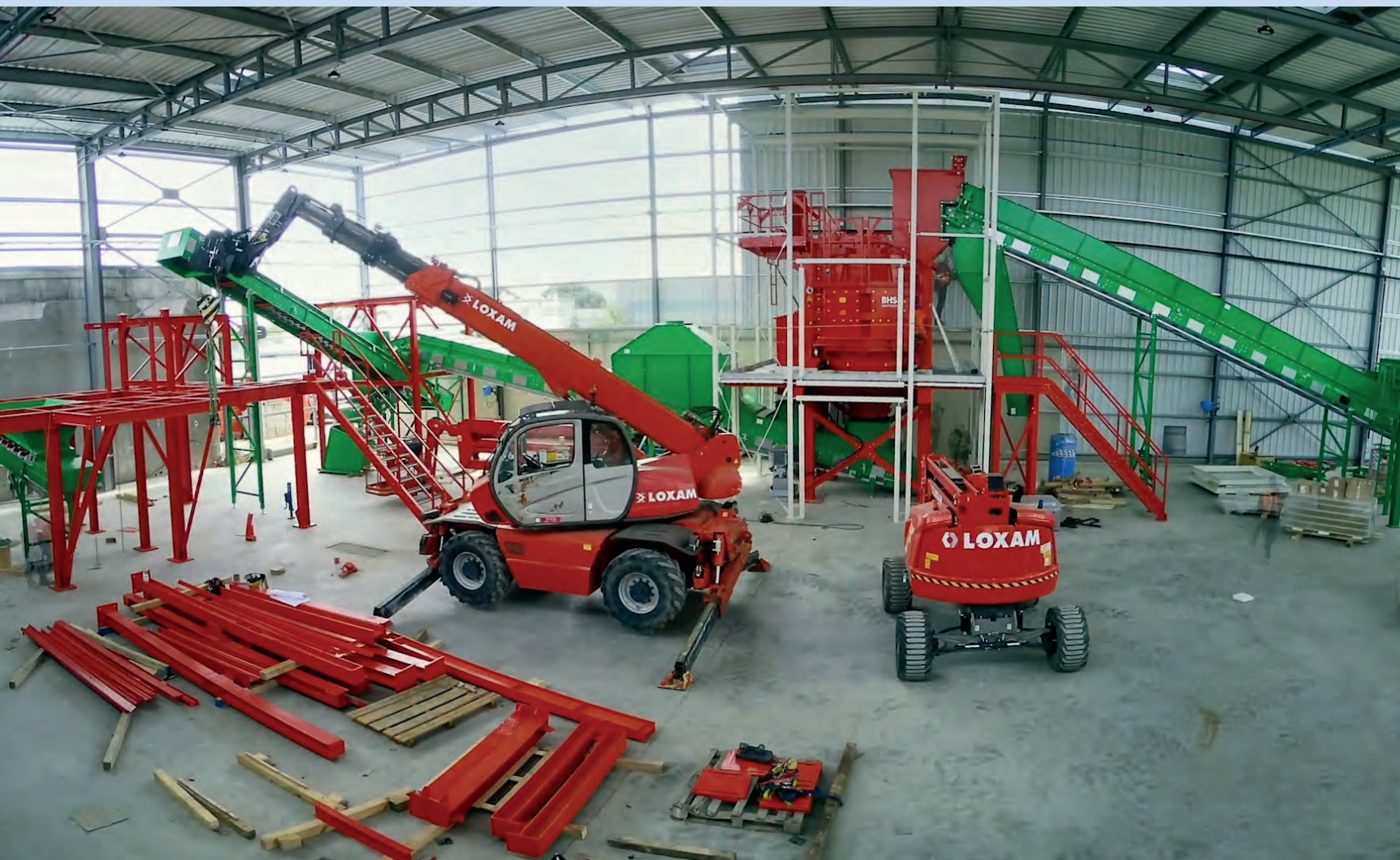
During the construction and assembly phase, the BHS Rotorshredder (type RS) can be seen in the background inside its noise protection housing.
