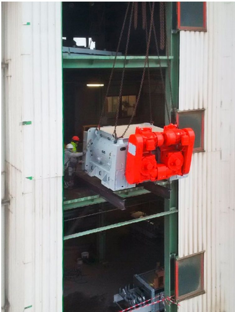
Installation of a new DMX 2600 Dry Powder Batch Mixer with dual flaps to modernize an existing dry powder factory.
